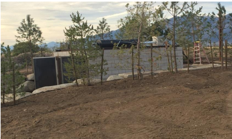
Photo 3: Shows Genoa Tree's stationary block kiln in Minden. The kiln is near completion and can process up to 9 cords of chips or whole wood per burn once complete.
