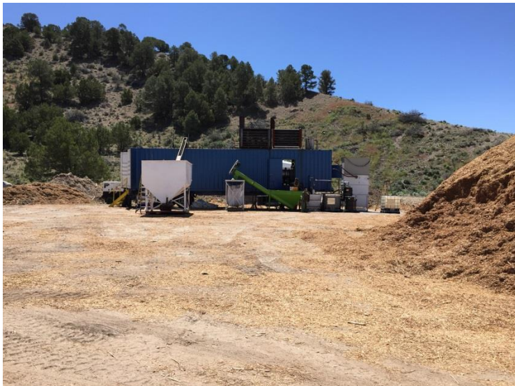
Photo 1a: Shows Amaron Energy's rotary kiln in Eureka. The kiln is housed inside the large shipping container, and is fed by the white chip feed bin and conveyor on the left. Finished biochar is emptied from the kiln into the green finished char bin and conveyor in the center, cooled with a water spray, and dumped into super sacks for storage and transportation. The equipment to the right of the finished char bin includes an incinerator and waste oil container.
